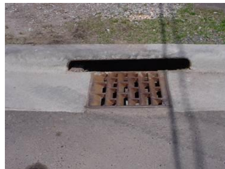
Storm Sewer - Catch Basin
